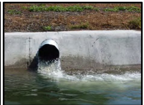
Substantial: steady stream with depth
