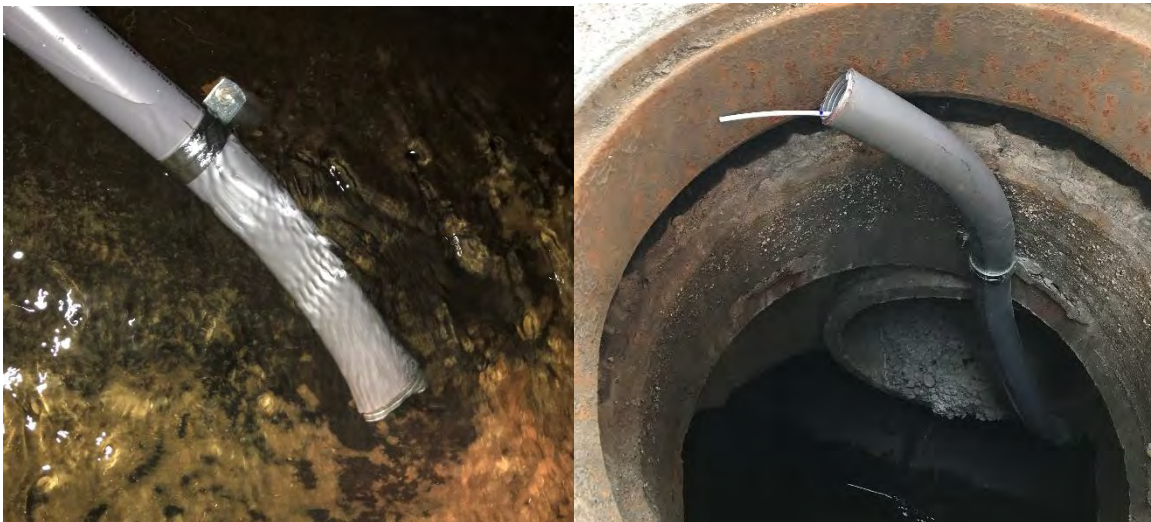
Figure 1. Installation of level loggers. Pictured left to right: conduit installation for loggers within stormdrain pipe with pinched end located at bottom of pipe; conduit installation with fiberglass rod extending from conduit for easy removal/replacement of level logger for download.
